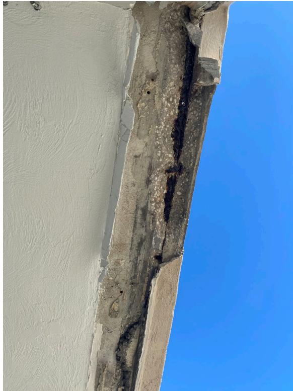
Picture 2: Unit 406 header spall
