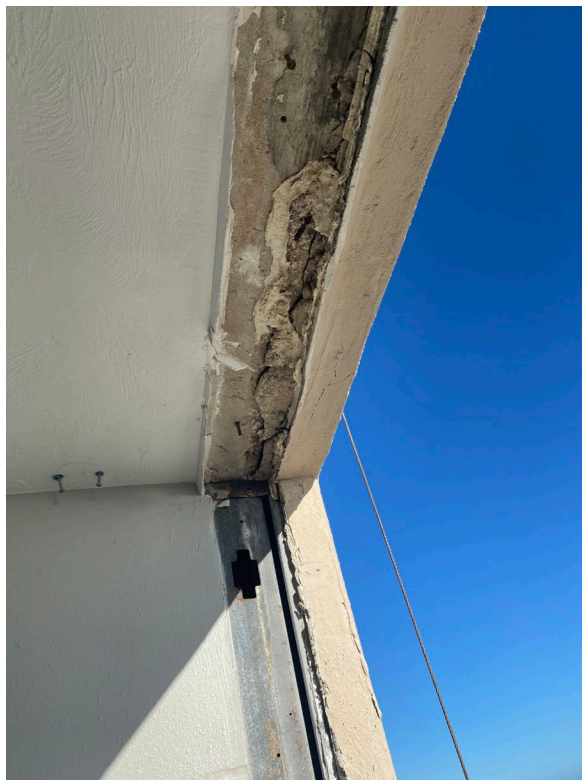
Picture 3: Unit 406 header spall
